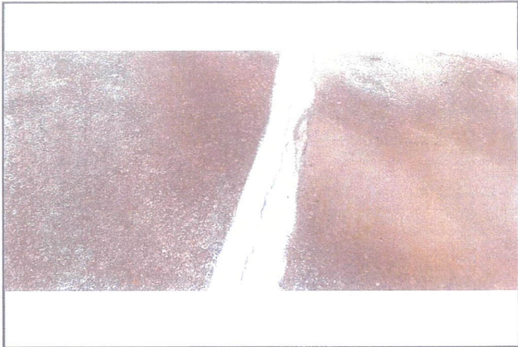
PHOTO No19 -Roof screed joints to be properly maintained
