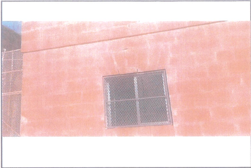
PHOTO No11 -External flat arches with disjointed voussoirs
