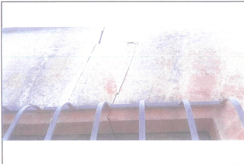
PHOTO NO 8 -Clear rotaional movement on flat arches on façade
