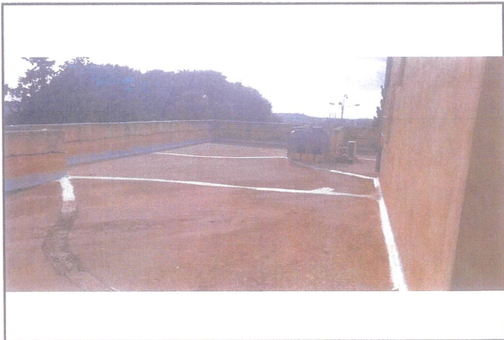
PHOTO NO. 20 - Screed joints especially those against parapet wall to be well maintained
