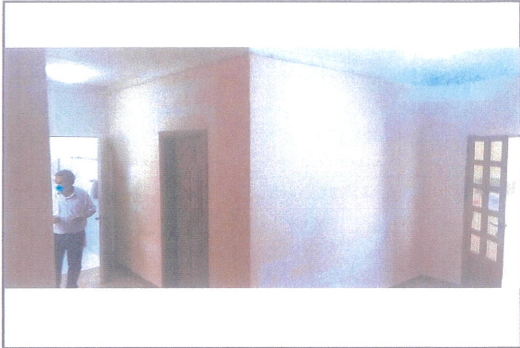
PHOTO No.7- Evidence of frequency of internal wall cracks
