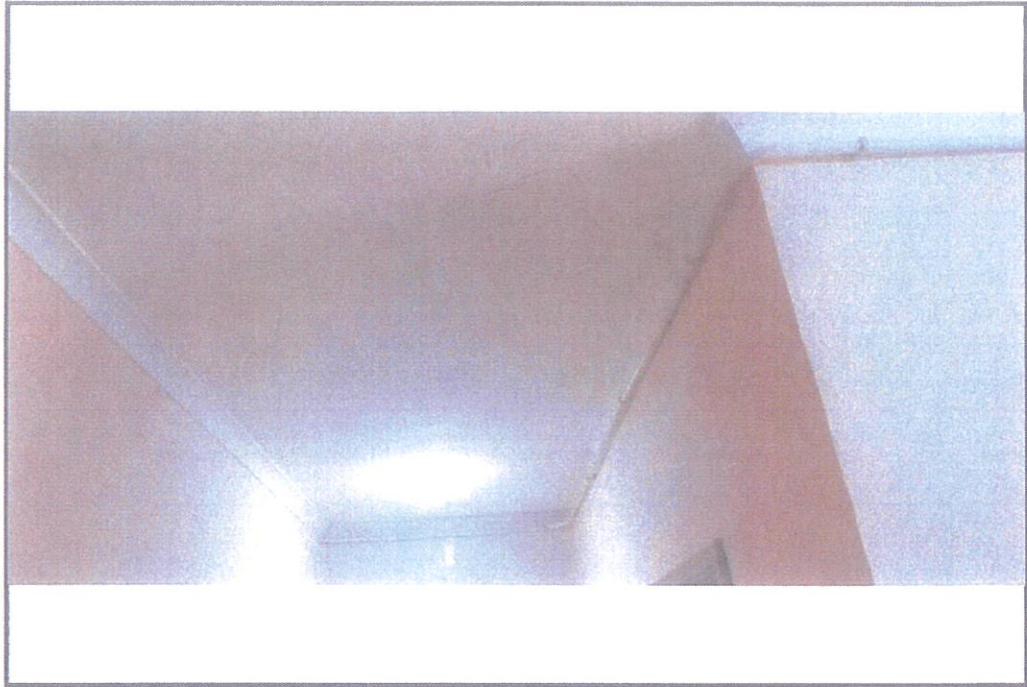
PHOTO No17 -Concrete Slab spalling defects over corridor
