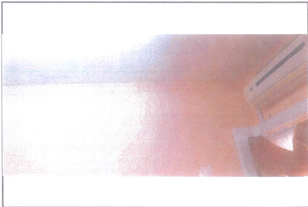
PHOTO NO 18 - Wall cracks and minor concrete slab spalling defects
