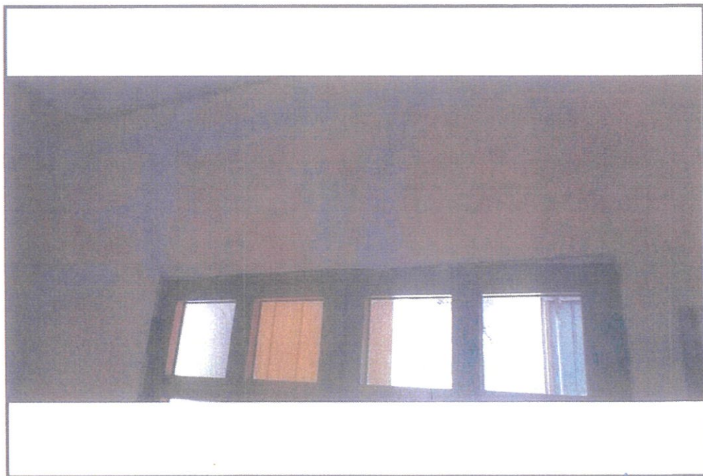
PHOTO NO.4--Wall cracks over main entrance flat arch plastered over
